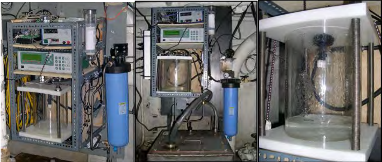
Figure 3.3. Seawater p\text{CO}_2 flow-through system in the forward engine room.
