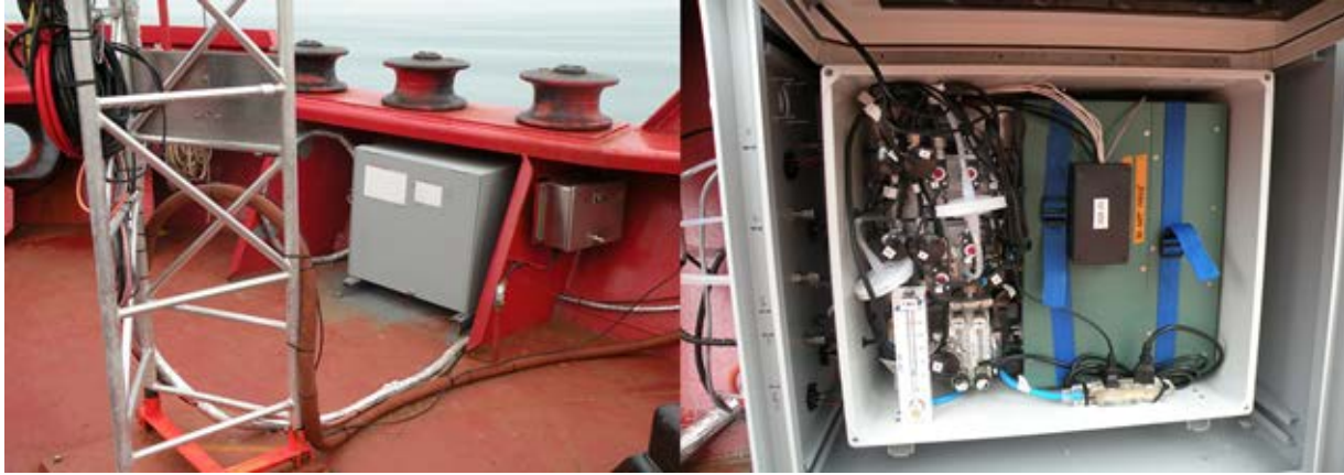
Figure 2.3. LI7000 gas analyzer enclosure at the base of the flux tower.
