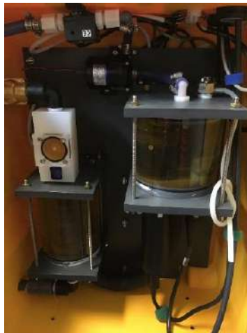
Figure 1-5 The underway optode / GTD (PIGI) system installed in the forward lab.
